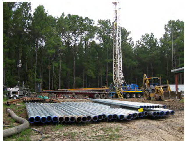
Figure 17. Drilling of the new monitoring well at Wee Tee State Forest in Williamsburg County (WIL-0355). The pipes seen in the foreground are sections of 6-inch and 4-inch diameter casing that were used to construct the 869-foot deep well.
