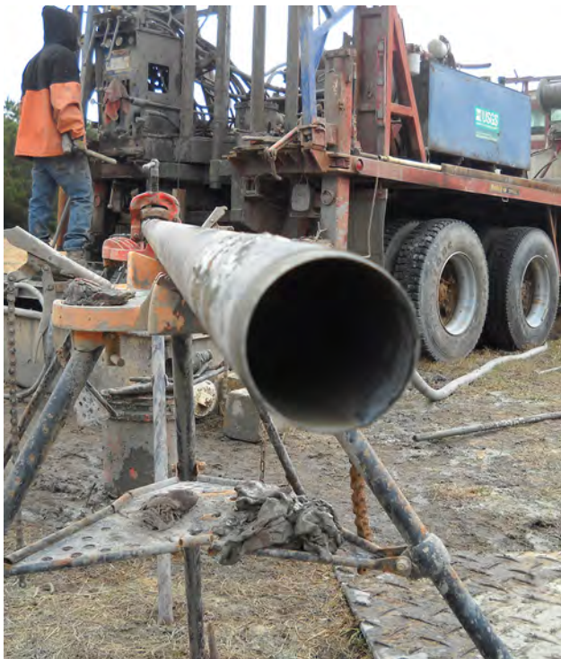
Figure 34. A view of the 2-inch diameter core barrel before it is lowered into the corehole at the Hobcaw site.
