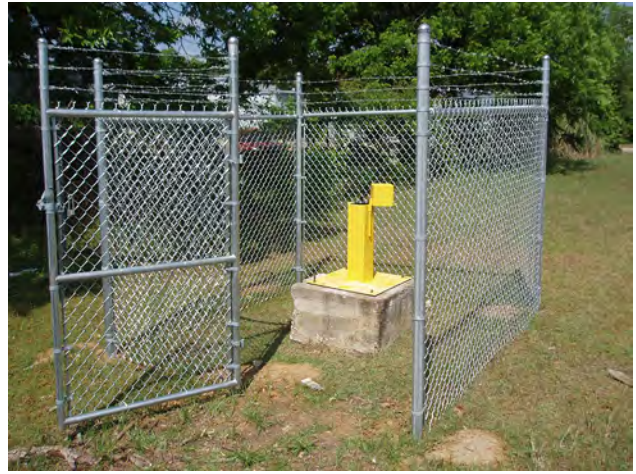
Figure 25. The Williston well (BRN-0078) site, after the new wellhead and fence were constructed.
