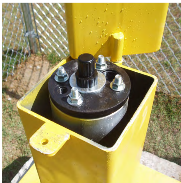
Figure 8. Pressure transducer ADR installation in a monitoring well (BRN-0078) in Williston, SC.
