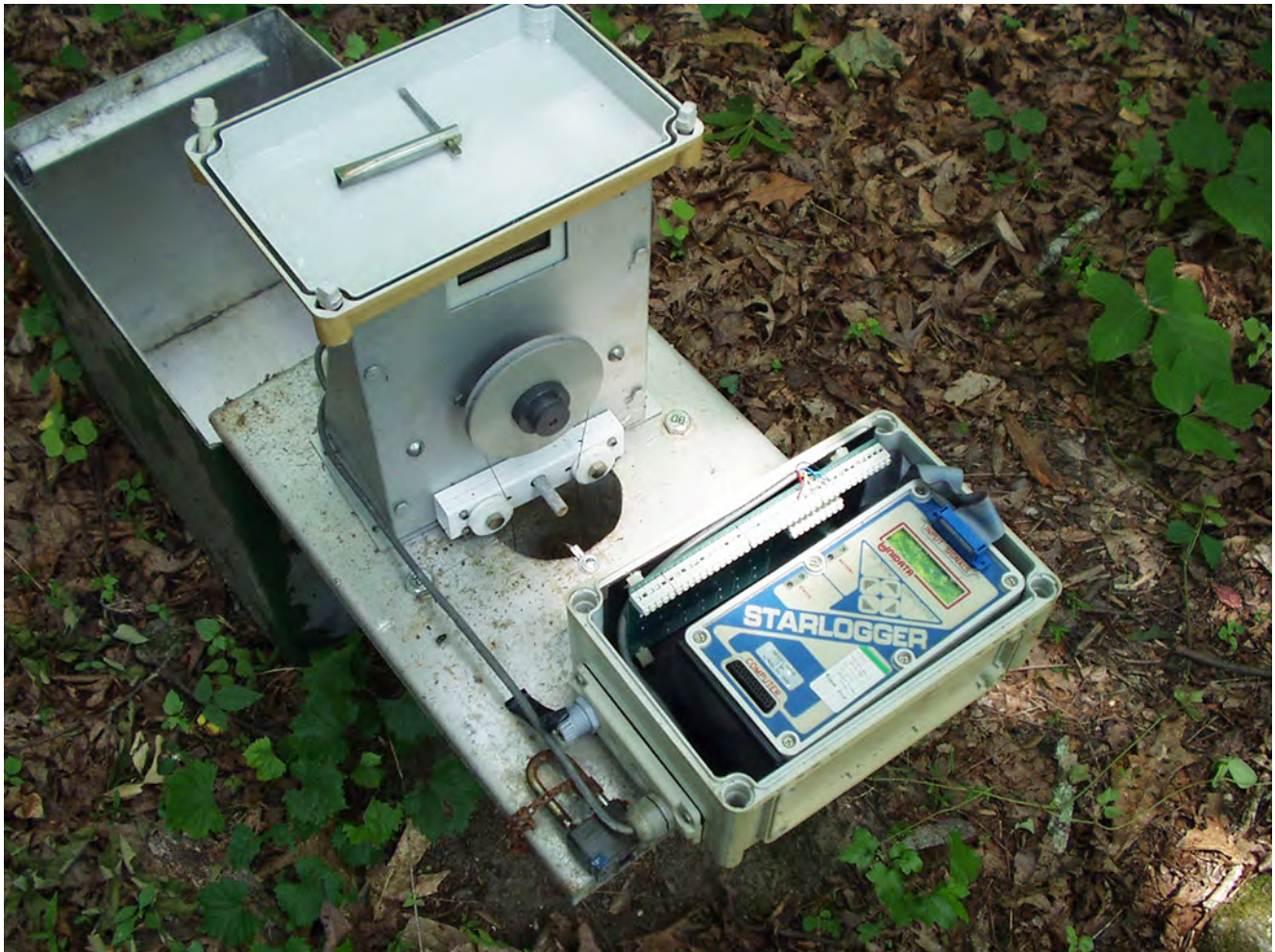
Figure 6. Shaft encoder water-level monitoring system installed in a well in Greenville County.
