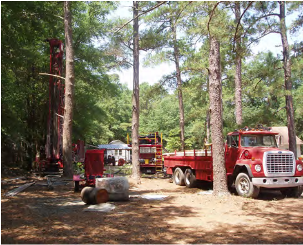
Figure 15. Drilling of the new wells at the Lee State Park cluster site in June 2012.
