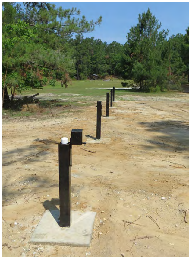
Figure 27. The five new monitoring wells constructed at Little Pee Dee State Park in June 2014.
