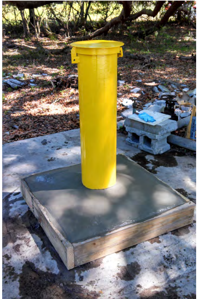
Figure 31. The new steel housing and concrete pad constructed for the Dixie Plantation well (CHN-0989).
