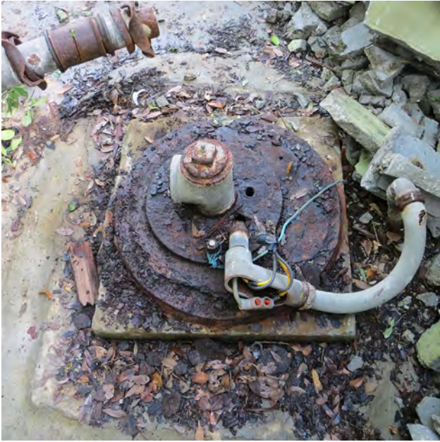
Figure 28. A view of the Dixie Plantation well (CHN-0989) in August 2013, before the old pump was removed and the well rehabilitated.
