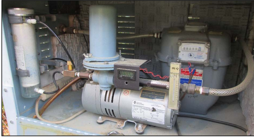
Inside View of Air Monitoring Station
