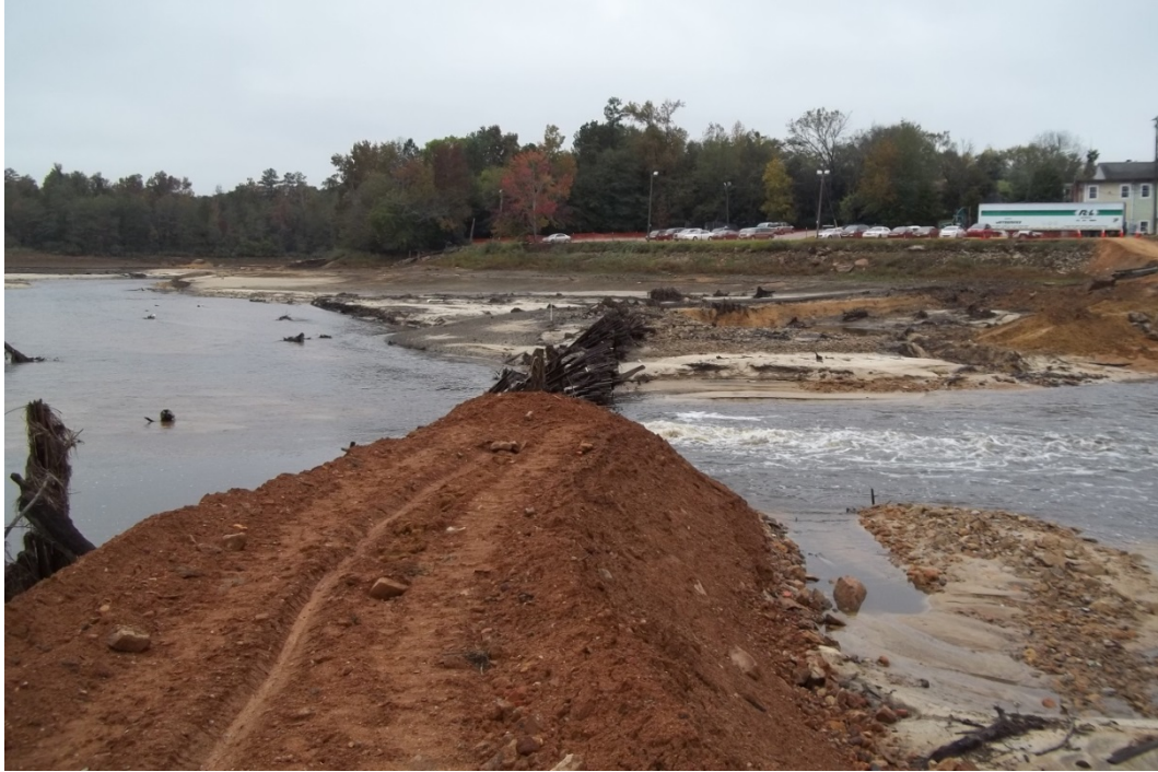
Photo 7: View showing newly placed earthfill and old timber cribbing upstream of the dam breach as viewed from the right abutment.
