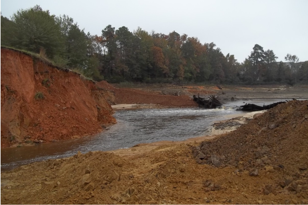
Photo 17: View is at upstream face of dam breach viewed from left abutment.
