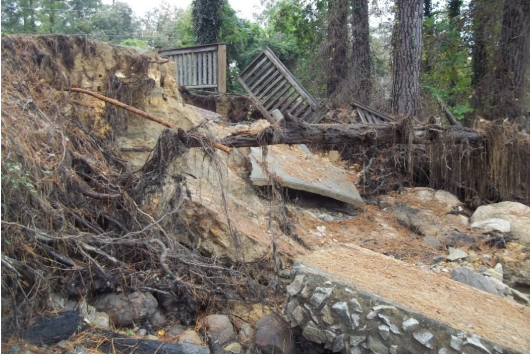
Photo 3: Remnants of wood walkway on left abutment.
