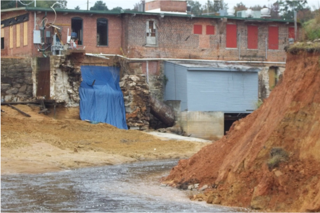
Photo 11: View is looking at penstock pipe.
