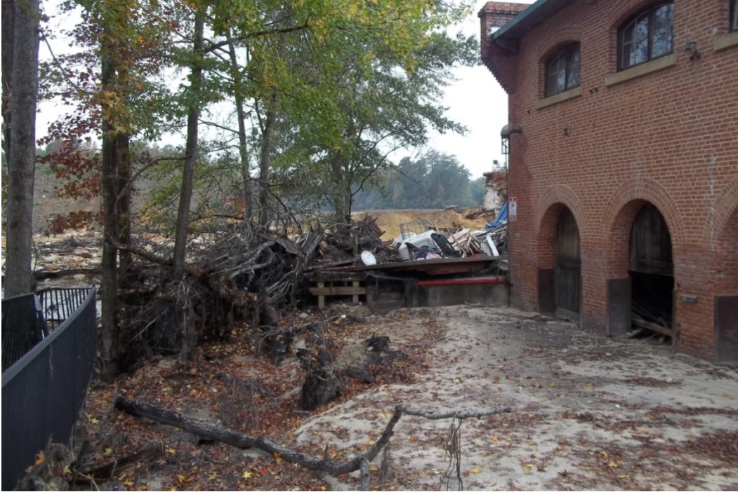
Photo 1: View shows left downstream abutment debris.
