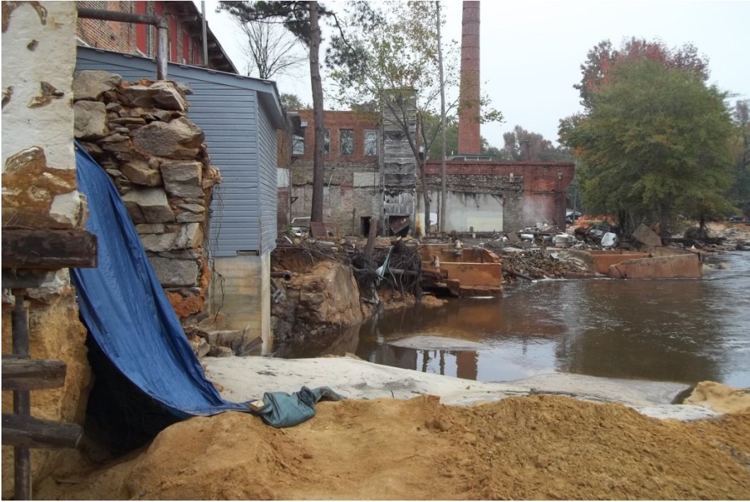
Photo 20: View is looking downstream at dam breach.
