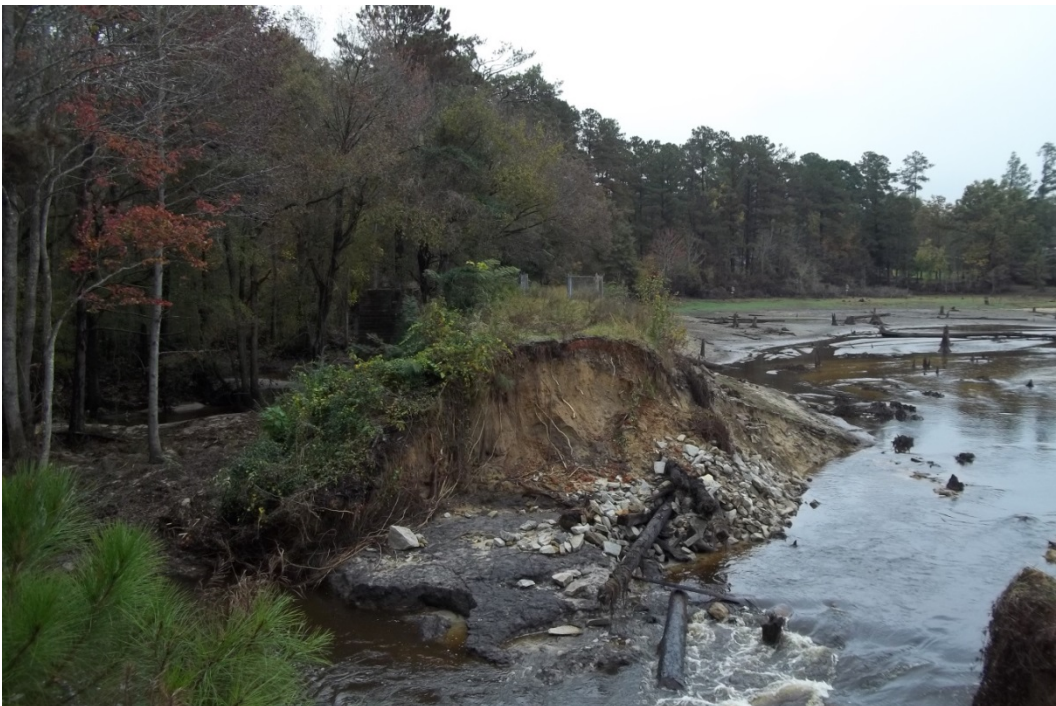
Photo 2: View is of center embankment at breach.
