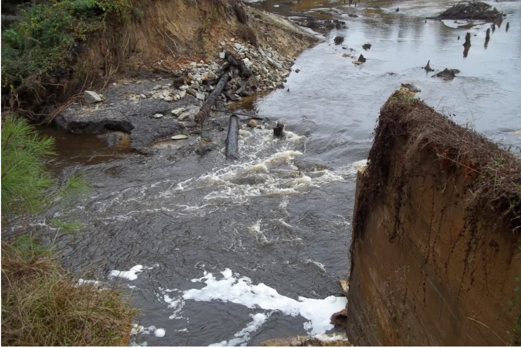
Photo 5: Looking at breach at right abutment.
