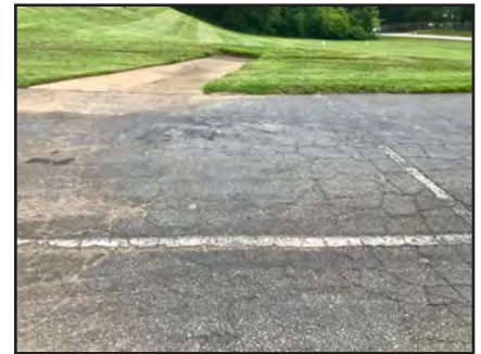
Parking lots that are directly connected to a storm drain, like this one here, can lead to heated runoff entering waterways.
